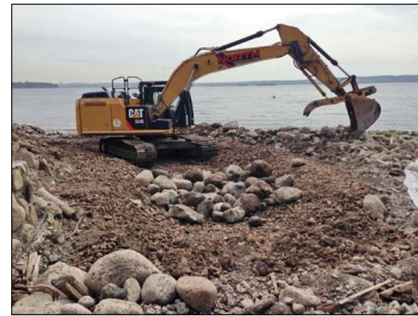
Image 4. Placement of stream armour rock to help prevent channel erosion by creek flow and waves.
